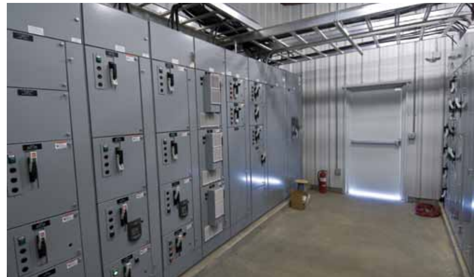
Heatec also provided and built the motor control center for the new emulsion plant. Photo courtesy of Heatec.
