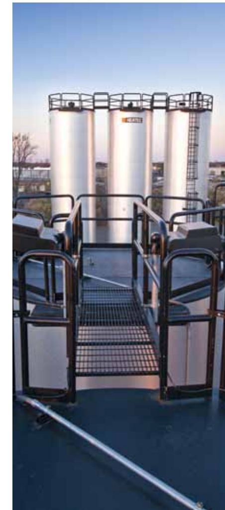
BCI Materials built in room for growth at their Charlotte, N.C., emulsion plant. Photo courtesy of Heatec.system.
