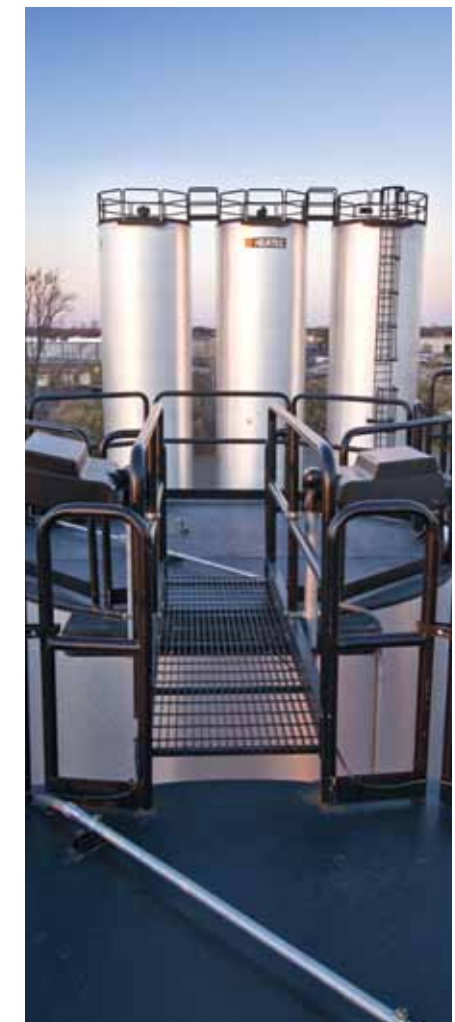
BCI Materials built in room for growth at their Charlotte, N.C., emulsion plant. Photo courtesy of Heatec.system.
